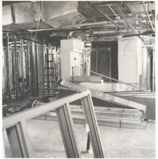
IT MAY NOT look like it, but this is now the Emergency Department reception area. The entrance and waiting room are out of the picture to the right.
