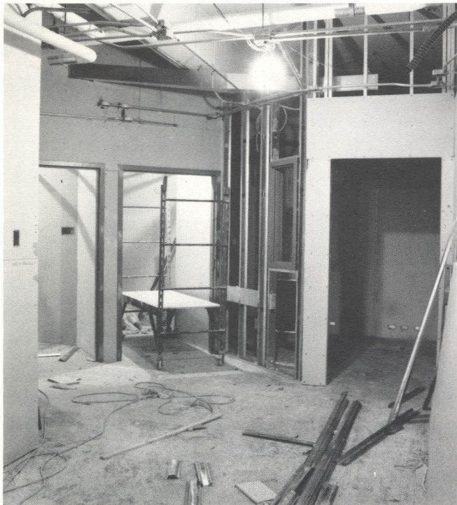
THE QUIET ROOMS and Psychiatry office are shown above. It is now March and the project is progressing as planned.
