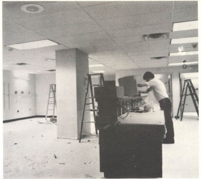
IN MAY, the computer terminal was installed at the nurses' station in the main exam room.
