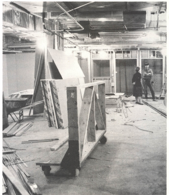
LOOKING PAST the future nurses' station, Emergency Department Administrative Director Karen Colby talks with a Murray carpenter. The rooms now have walls.
