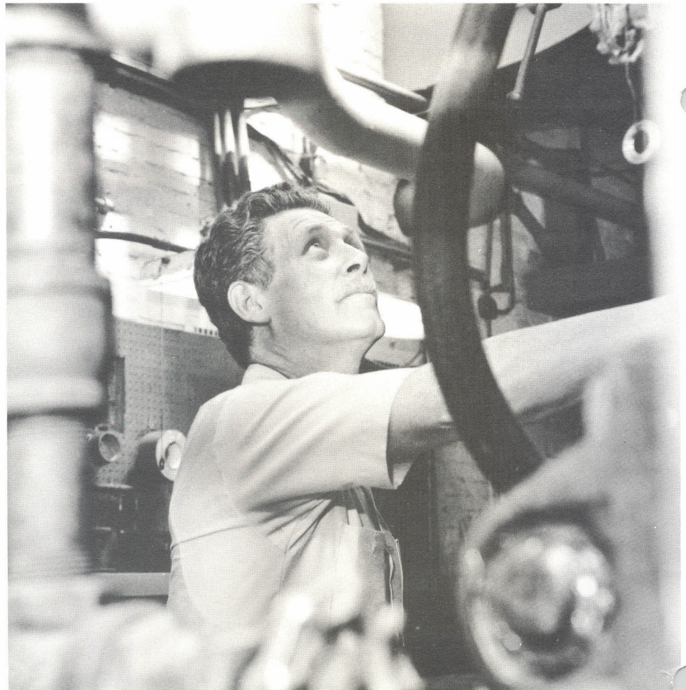
A REAL HOT SPOT is MMC's boiler room where temperatures reached 120 degrees this past week. Richard Doughty, BST adjusts the boiler controls during one of his hourly rounds.
