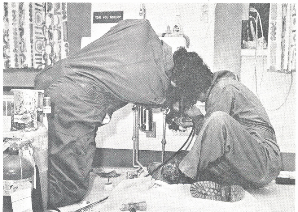
ONE OF THE THINGS "You Don't See" is the work involved in tracing and repairing a leaky pipe. This pipe was leaking behind a sink on pediatrics, but the water was showing up two floors down in the Outpatient Clinics. Plumbers Ray LeDoux (left) and Don Bernier of MMC's Engineering Services Department found the leak and fixed it. (A/V Photo)
