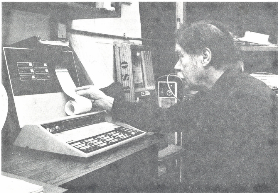
HARDY NORRIS receives a printout from the Delta 1000 in Operational Maintenance, one part of the energy management program at Maine Medical Center. The computer monitors temperatures, relative humidity, gas and water pressure, and heating and cooling activity throughout the MMC complex. (A/V Photo)
