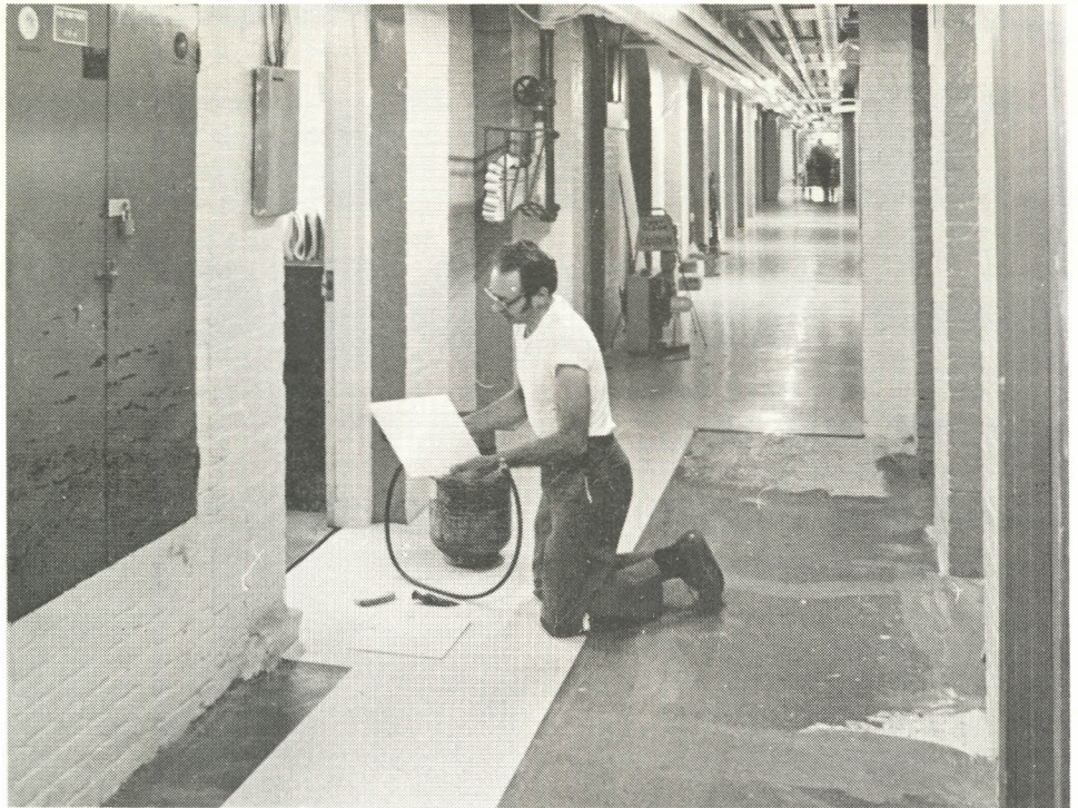
THE GROUND FLOOR CORRIDOR OF THE 1870 MAINE GENERAL BUILDING has a new look these days, having been tiled from end to end. The entire job -- down the hall, around corners into recesses, around fixtures -- took over 3,000 individual tiles. Tile installer Sanford F. Fuller, Sr., is shown above nearing the end of the road. (A/V Photo).
